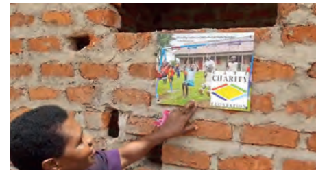
Christian Childcare Programme: construction of 4 houses for the teachers of the primary school of CCP in Uganda.
